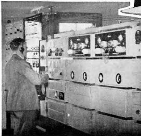
Monitoring the Anglo-Australian Wireless Telephone Channel at A.W.A. Receiving Centre, La Perouse.
