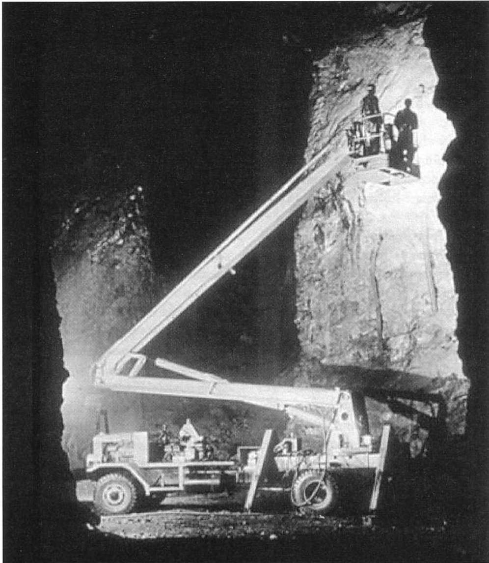
Scaling loose rock in the Friedensville Mine, ca. 1976. (Courtesy of Ken Cox.)
