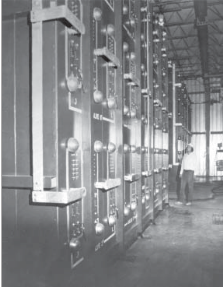
Figure 7. Banks of General Electric thyristors used at a converter station in Stegall, New Hampshire.
